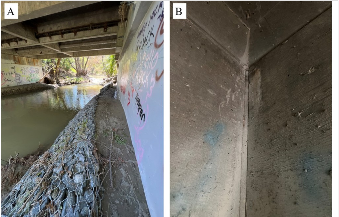
Figure 23. (A) San Ramon Creek Bridge – Structure ID 28 C0391. Substructure of structure ID 28 C0391 facility over San Ramon Creek in Contra Costa County, California, USA. (B) San Ramon Creek Bridge – Structure ID 28 C0391. Guano staining in a corner joint of structure ID 28 C0391 facility over San Ramon Creek in Contra Costa County, California, USA.
